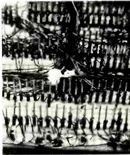
HOLDING WIRE-WRAP POSTS in place with hot-melt glue. A wire run is also held down with the glue. If you see a leaning post here, that's because it was either glued that way or the post is bent. These glued-down posts hold resistors and transistors.
